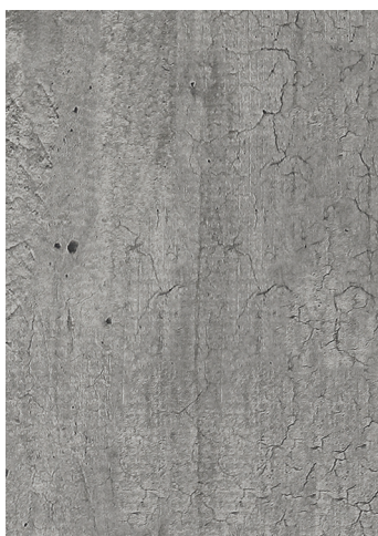
2005 CEM Cracked Cement
